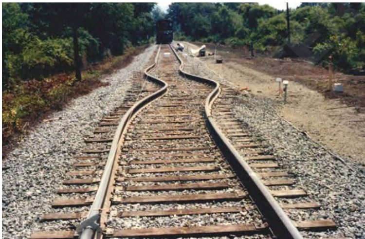
Figure 7.15-7: Example of Rail Buckle from Extreme Heat
